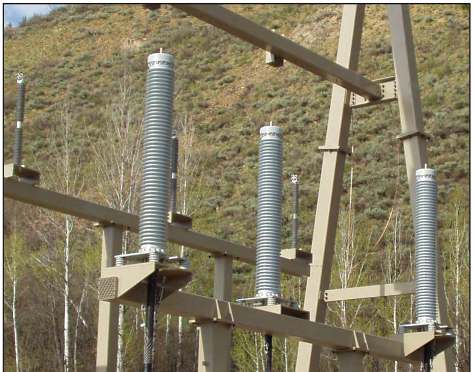
▲ G&W 245kV terminations with composite insulators.
