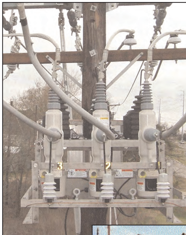
Figure 1 above: Pole mounted, 15kV Viper-ST recloser.
