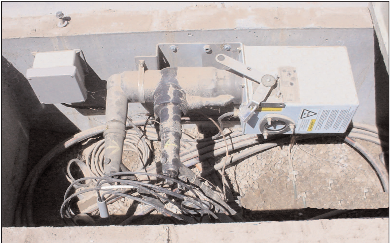
G&W's 15kV, 200A solid dielectric switch minimized the vault size requirement and offered convenient access to the manual trip handle for easy hookstick operation from above ground.
