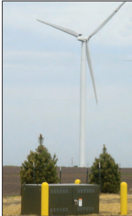
▲ Padmount switch in a collector system.
