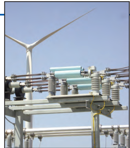
▲ Substation mounted 38kV CLiP
