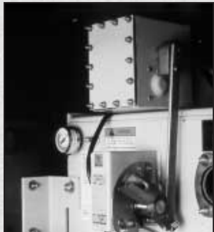
Top mounted motor actuator on a SF6 gas switch.
