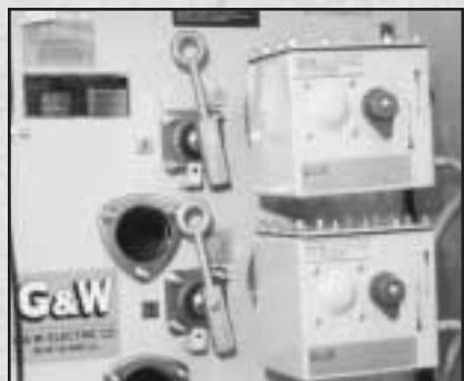
Front mounted actuator with cock-and-trip mechanism on an SF6 switch.
