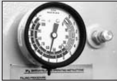
▲ Pressure gauge and fill valve
