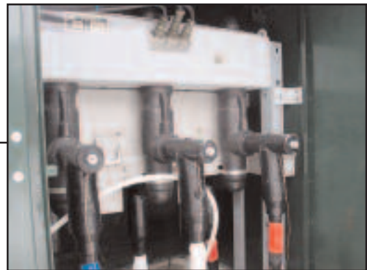
Photo (right) shows a front/back configuration using Z modules.
