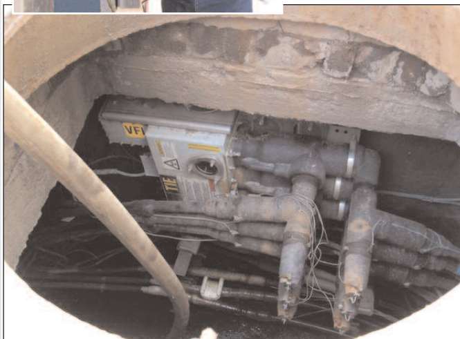
Three phase fault interrupter mounted horizontally due to limited vault space. The vault opening is only 23" in diameter.
