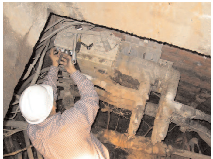
Vaults are subject to complete submersion.
