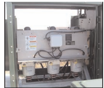
Recloser operator compartment.
