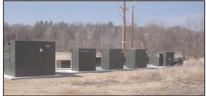
The padmount solution includes a three phase transformer (left), voltage regulators, Viper -ST recloser and numerous single phase switches.
