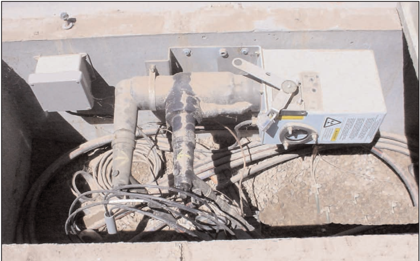
G&W's 15kV, 200A solid dielectric switch minimized the vault size requirement and offered convenient access to the manual trip handle for easy hookstick operation from above ground.
