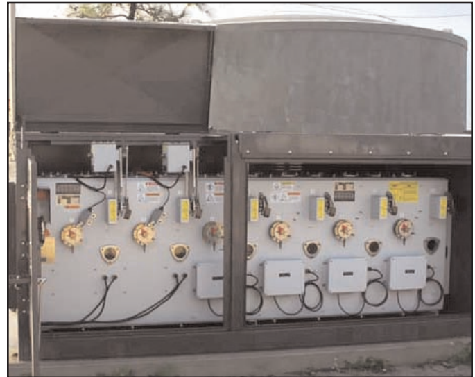
Six way padmount switch with motor actuators on source ways 1 and 2.
