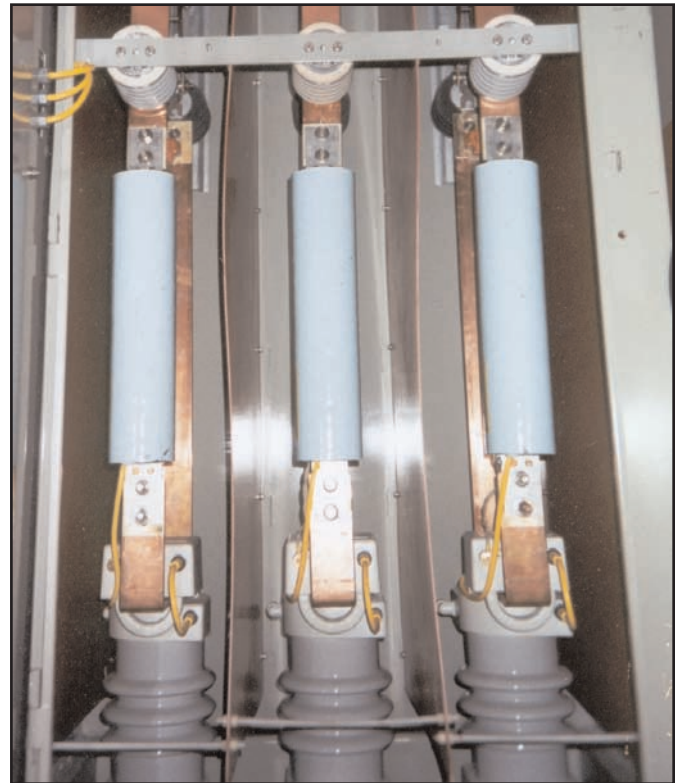
▲ G&W 15kV CLiP fuses mounted in an enclosure.
