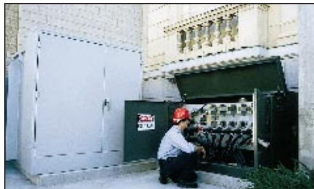
Fig. 6. Pad-mounted switch (G&W Electric Co.) incorporating two source feeders and two vacuum interrupter protected taps.
