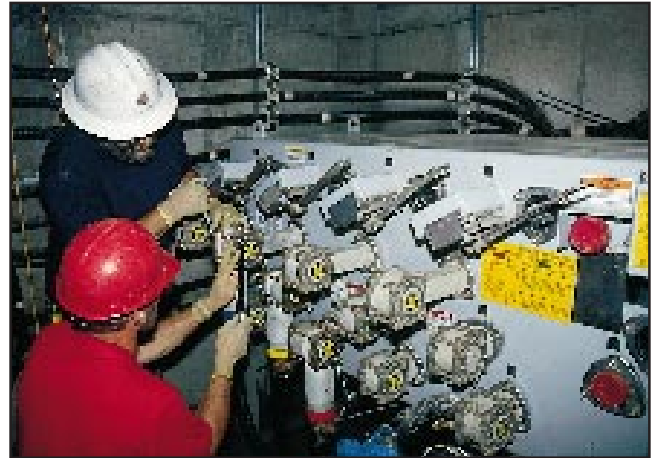
Fig. 8. Cable ends bolt to mating switchgear entrance bushings.
