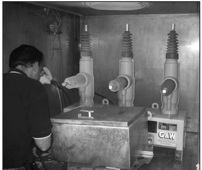
▲ G&W Viper-S recloser including SEL 351-R control within a sealed, cold temperature chamber prior to testing.
