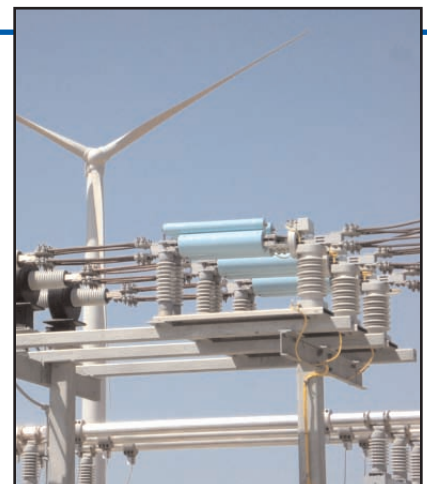
▲ Substation mounted 38kV CLiP
