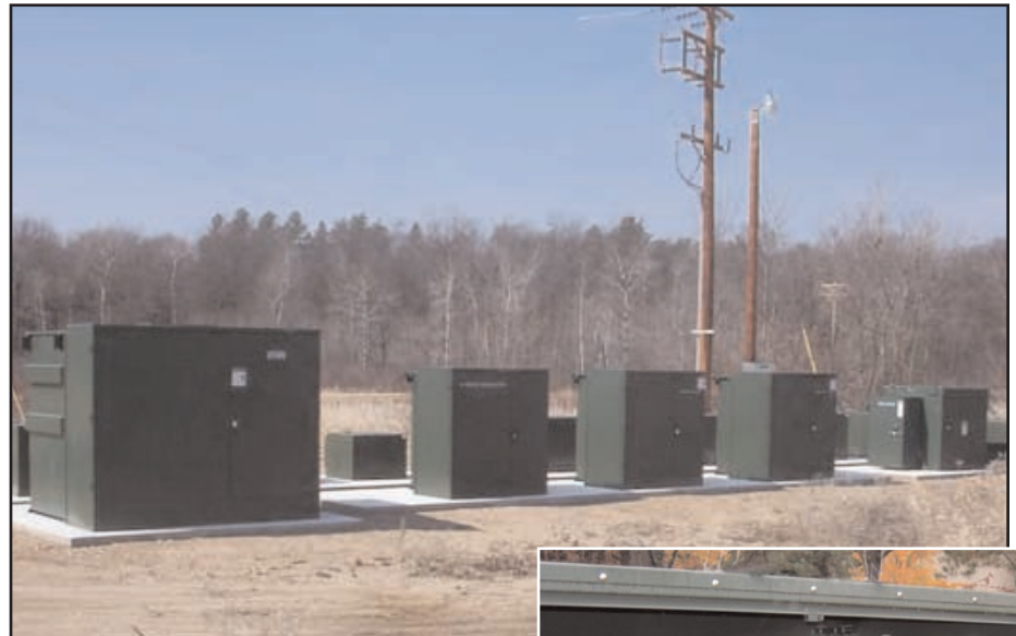
▲ Multiple padmount switches in a collector system.
