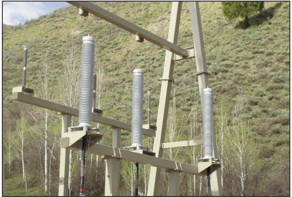
▲ G&W 245kV terminations with composite insulators
