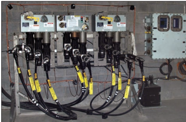
▲ Three-way, solid dielectric, automatic transfer switch with submersible control cabinet and potential transformers.
