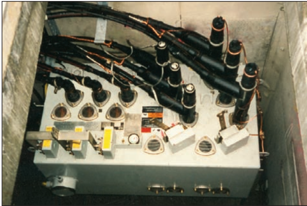
▲ Subsurface load and fault interrupting switch with top mounted operators for above ground operation.
