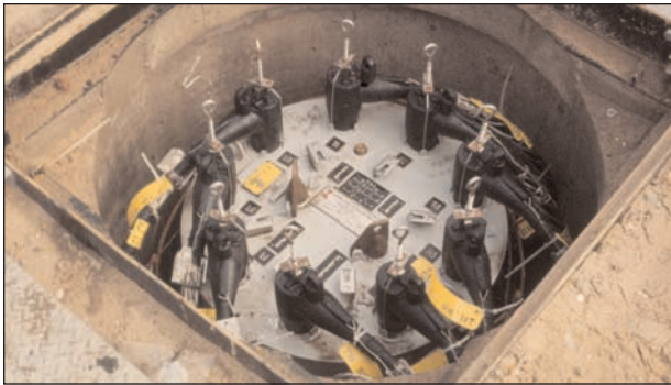
▲ Round subsurface switch within a confined vault.
