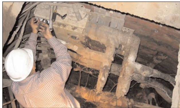
▲ Automated solid dielectric switch after numerous total submersions.
