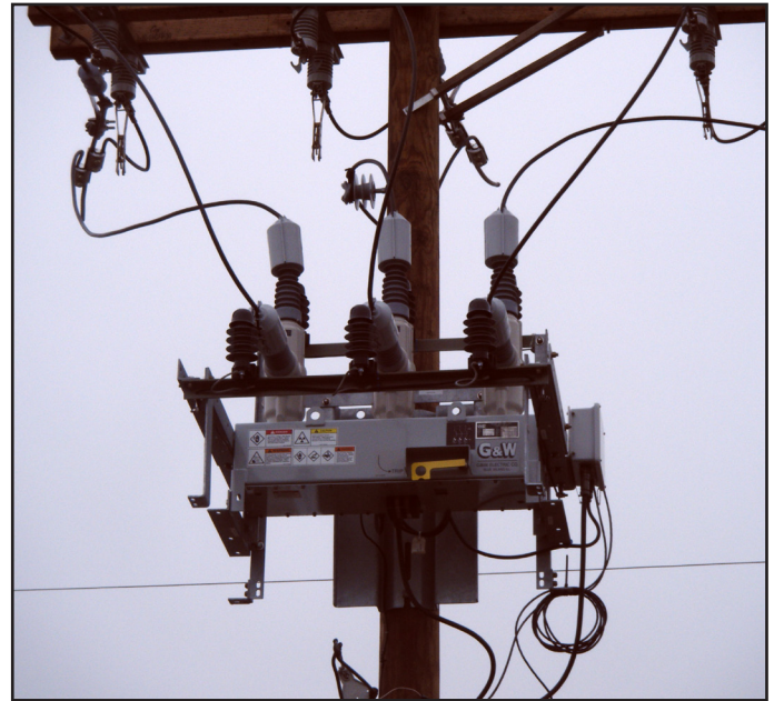
15kV Viper recloser with SEL 351-R control.
