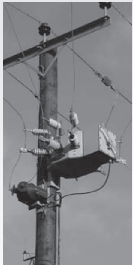
▲ 15kV, model RP switch with lightning arresters and potential transformers.
